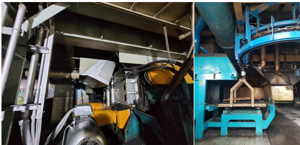
Figure 15. New suction points. Left: around VC, Right: between VC and pool.
